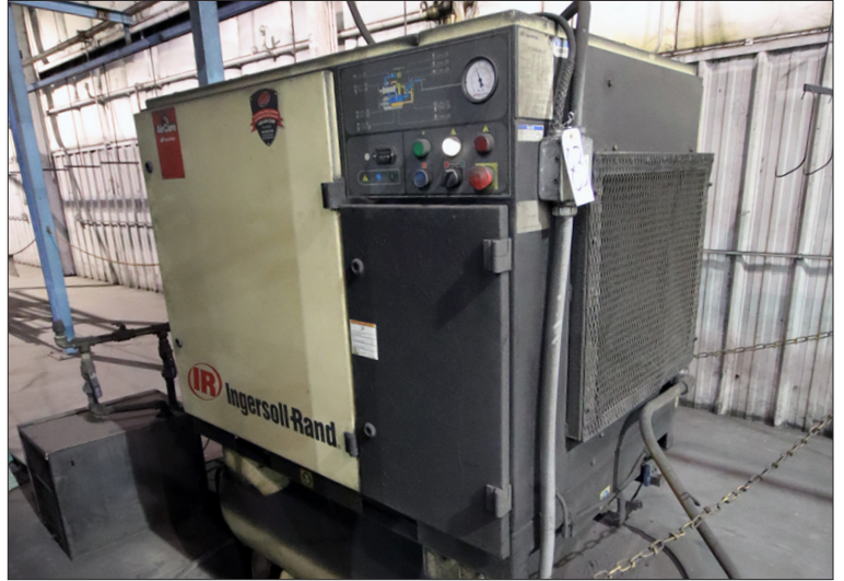
Ingersoll Rand SSR-UP6-25-125 12 Air Compressor
